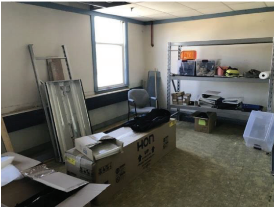
Interior view - storage area (some deferred maintenance evident)
