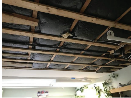
Interior view - deferred maintenance
